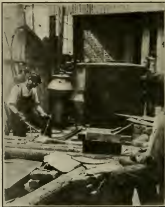
THE MILBURN CUT-WELD TORCH WELDING BLOW-HOLES IN HEAVY IRON RETORTS AT EDGEWOOD ARSENAL, THE LARGEST GAS PLANT IN THE WORLD.
